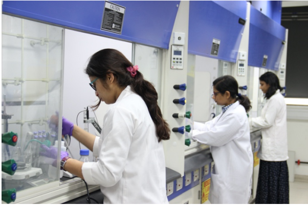
Wet Lab Fume Hoods for chemical work
